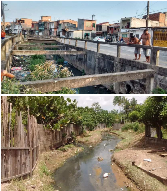
Figure 6 - Examples of sewage in Belém and Macapá
